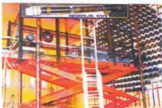
Fig.1 INGRES-2S system under operation at MAPS-1
